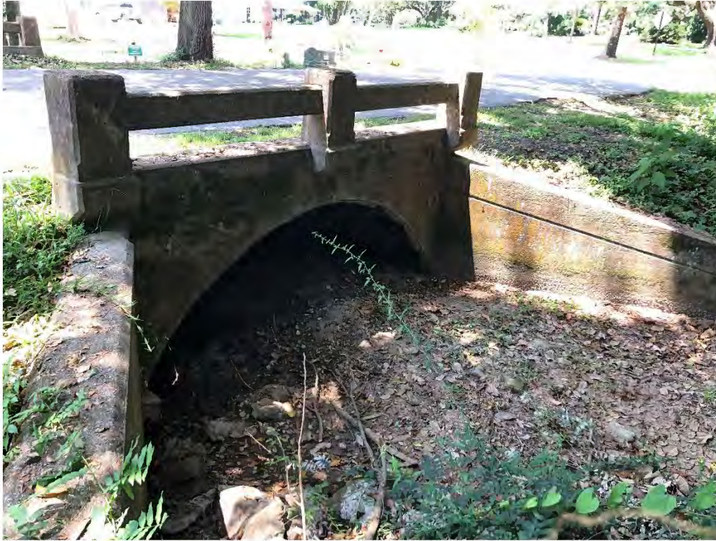
Figure 9671: Photo taken facing South toward a very silted OAK-CO-26 at the intersection of Oak St and a residential driveway.
