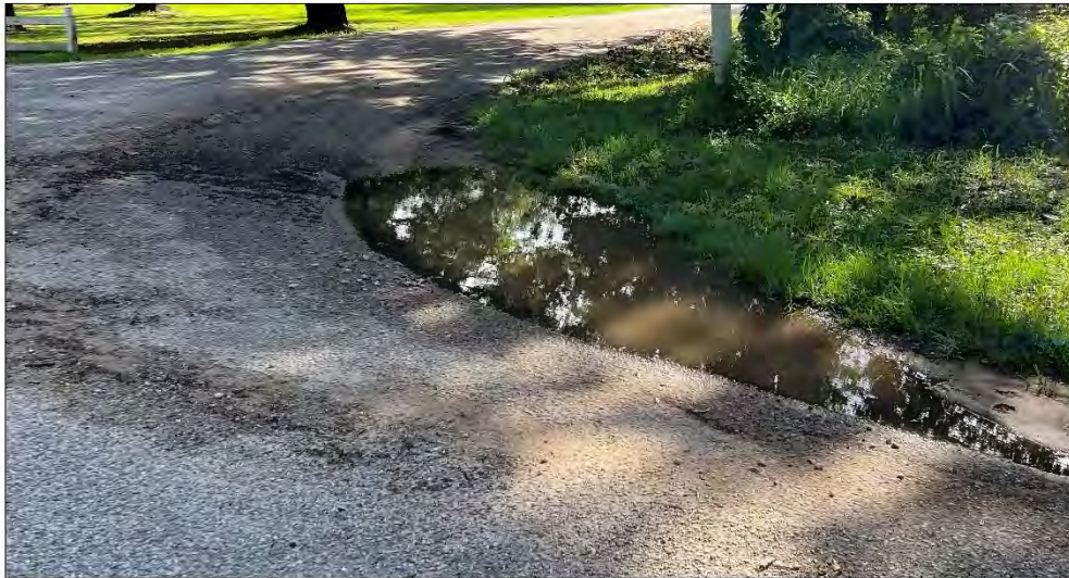
Figure 5. General view of standing water.
