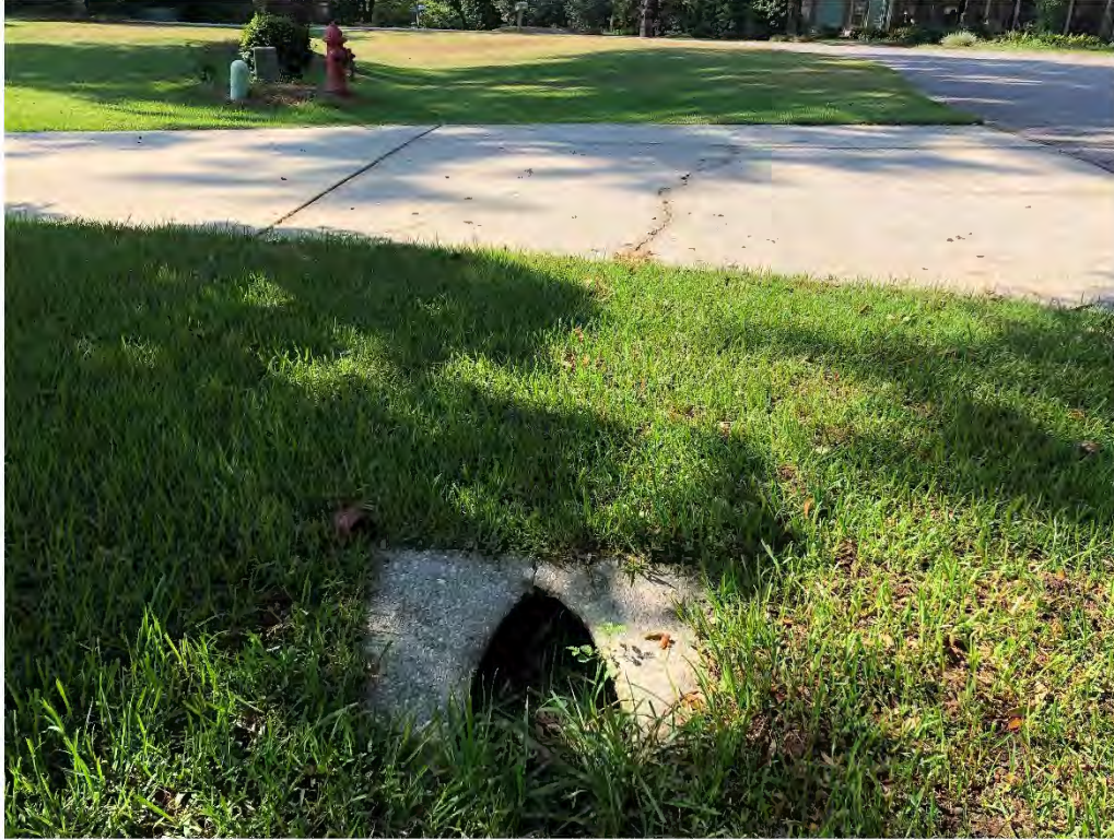
Figure 9486: Photo taken facing South toward VG-CO-2 at the intersection of Village Green Drive and a residential driveway.
