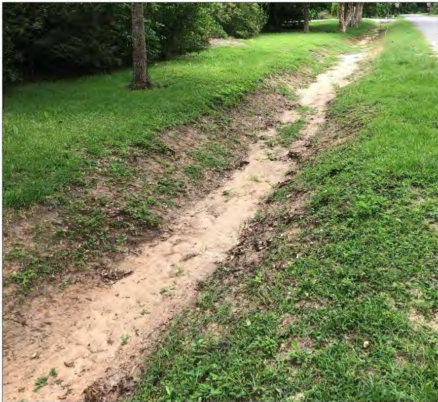
Figure 4. General view of eroding ditch.
