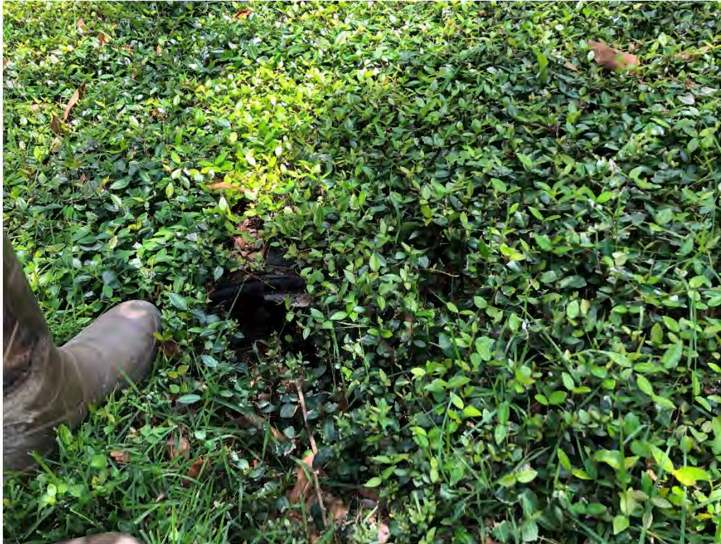
Figure 9088: Photo taken facing East toward an overgrown P-CO-26 along Oak St.
