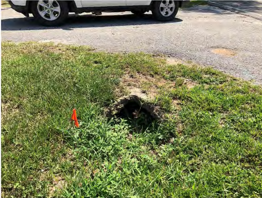
Figure 9572: Photo taken facing East of MN-CO-14 at the intersection of Gates Ave and a driveway.
