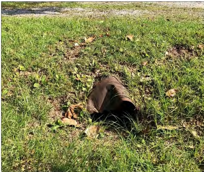
Figure 1. General view of a damaged culvert.
