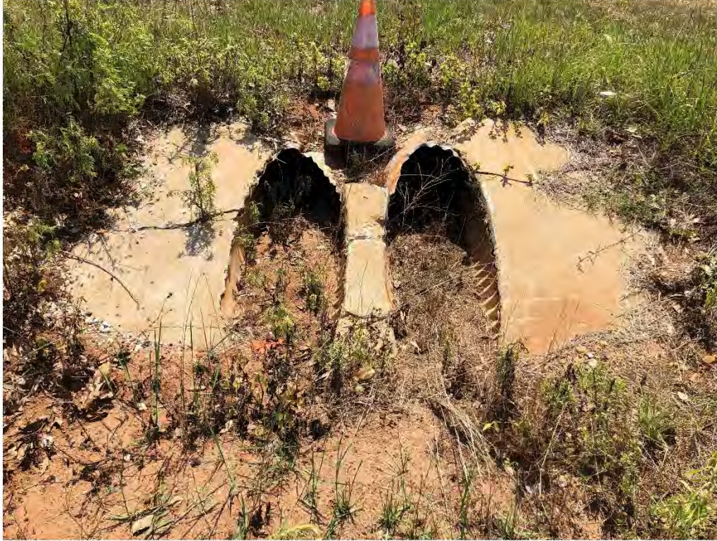
Figure 9617: Photo taken facing West toward a very silted pipe at the intersection HWY 98 and a driveway.
