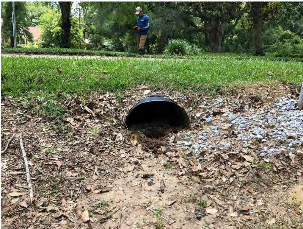
Figure 9089: Photo taken facing West toward a silted P-CO-26 along Oak St.
