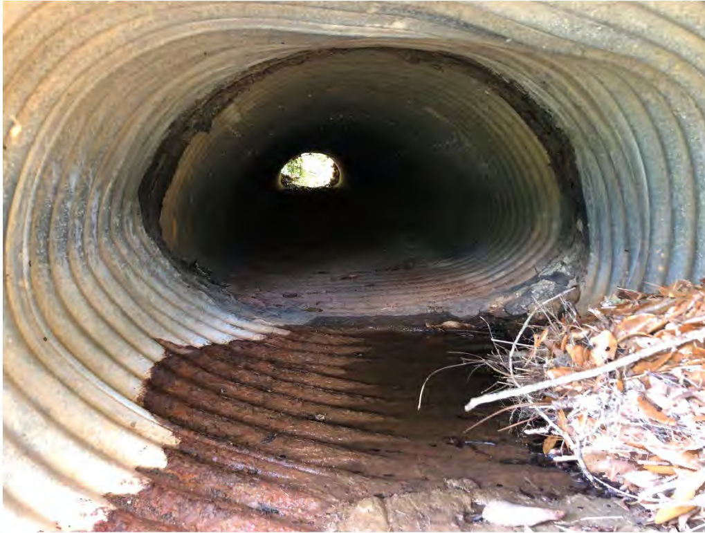
Figure 9112: Photo taken facing West toward a crushed corrugated metal P-CH-28 along Oak St.
