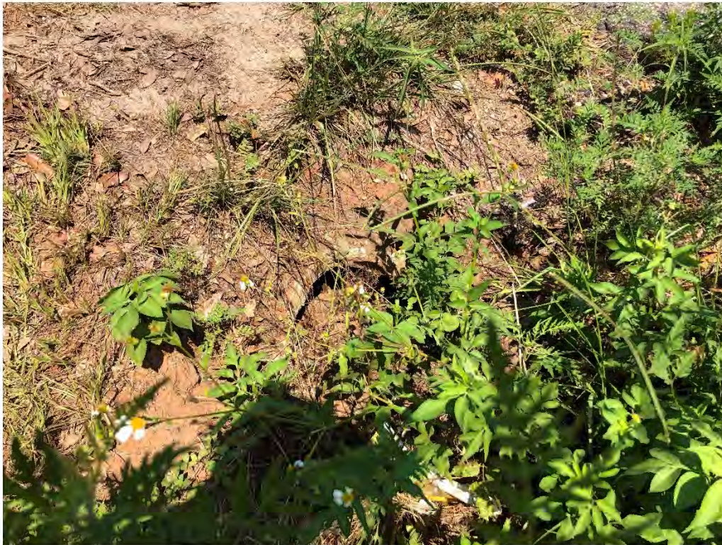
Figure 9616: Photo taken facing North toward a very silted pipe at the intersection HWY 98 and Schindler Ln.
