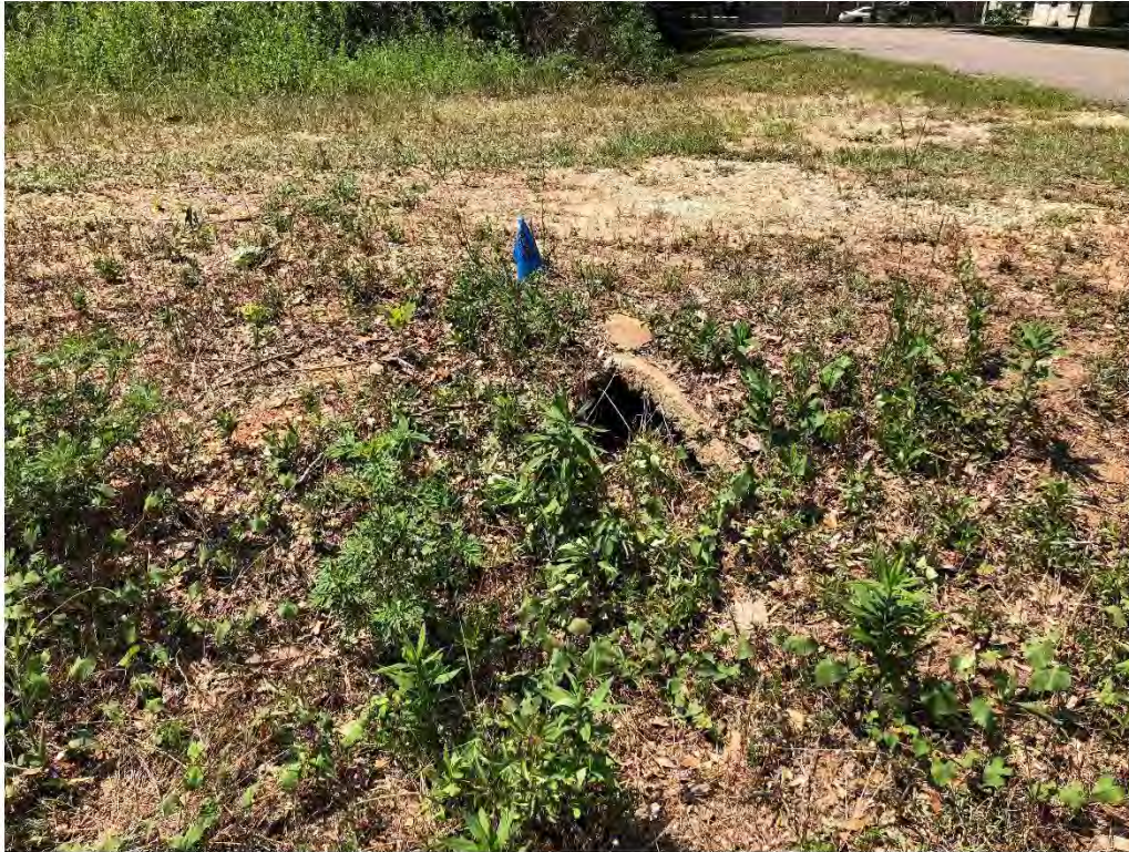
Figure 9623: Photo taken facing South toward a very silted OAK-CO-7 across Jessamine St.
