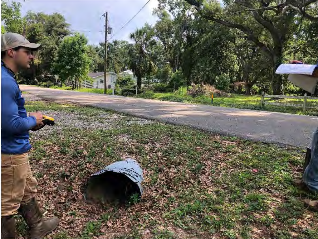
Figure 9240: Photo taken facing SW toward a silted P-CO-17 along Pecan Grove St.
