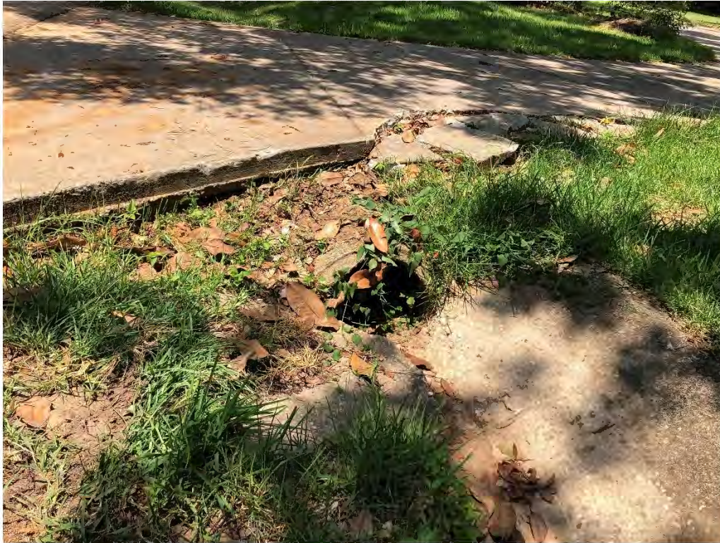
Figure 9661: Photo taken facing SW toward a concrete ditch that is full of dirt along Oak St.
