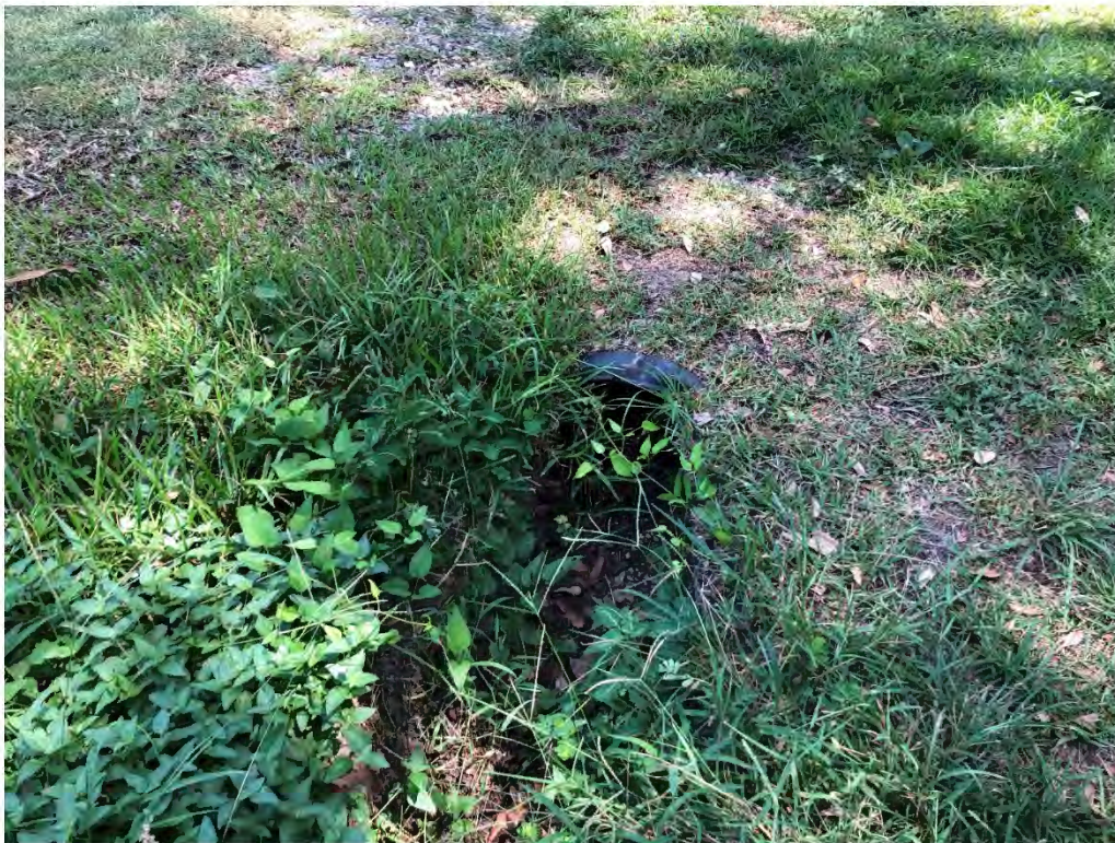
Figure 9604: Photo taken of a silted pipe at the intersection of School Street and a driveway.
