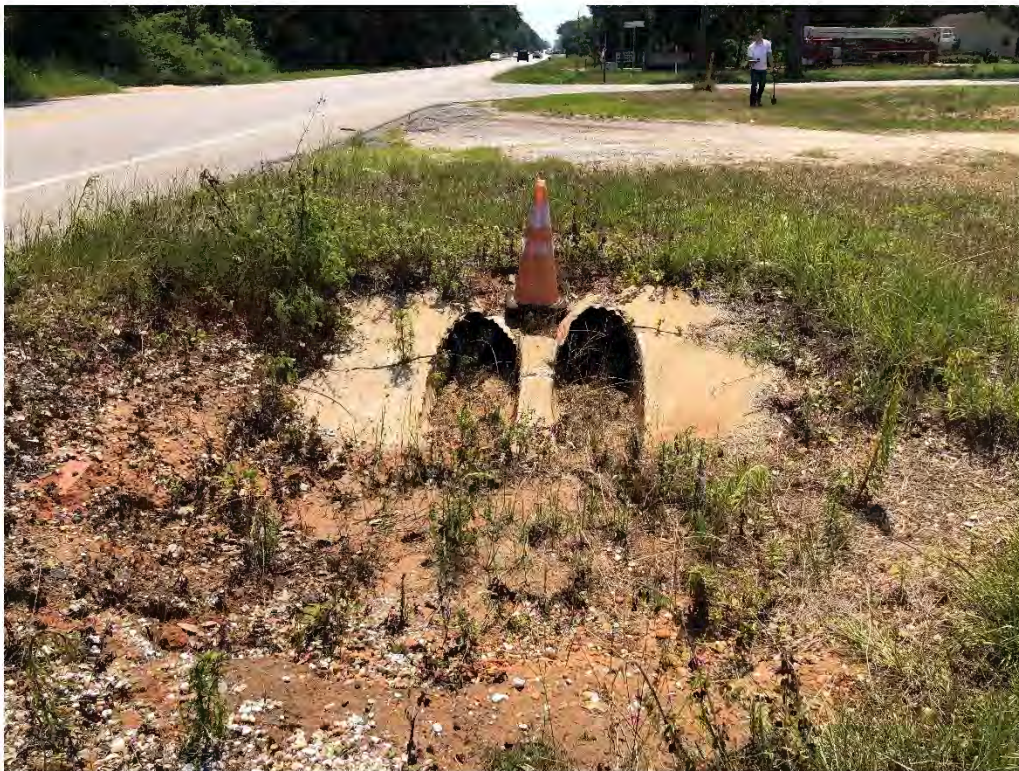
Figure 9618: Photo taken facing East toward a very silted pipe at the intersection HWY 98 and a driveway.
