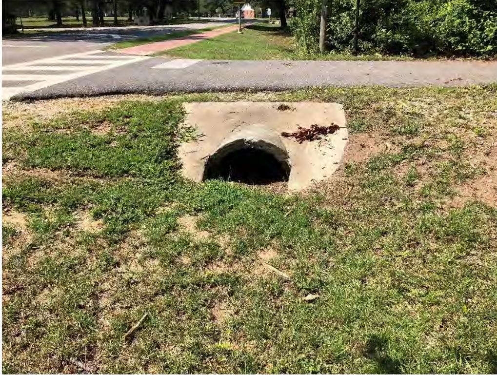
Figure 9546: Photo taken facing SE toward OAK-CO-31 at the intersection of HWY 49 and School Street.
