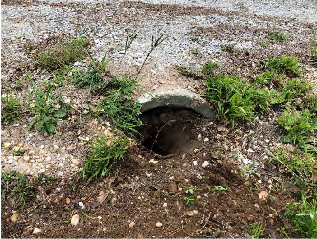
Figure 9096: Photo taken of a very silted P-CO-26 along Oak St.
