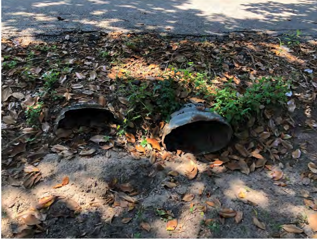
Figure 9599: Photo taken of a silted pipe at the intersection of School Street and Magnolia Ave.
