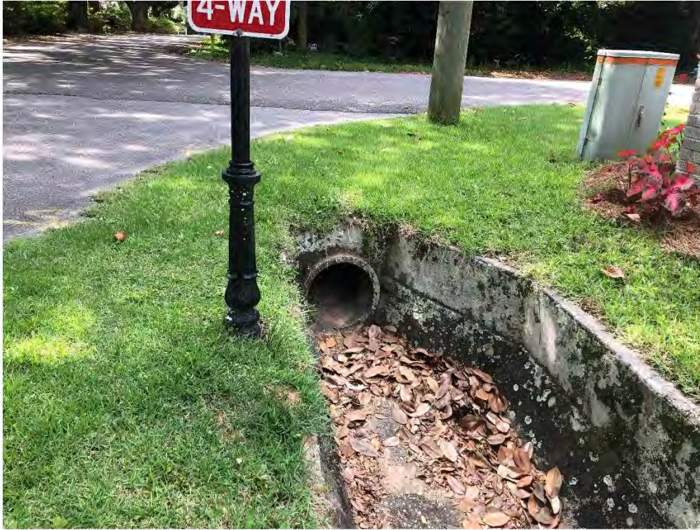
Figure 9228: Photo taken facing South toward J-CO-3 at the intersection of Oak St and Jessamine St.
