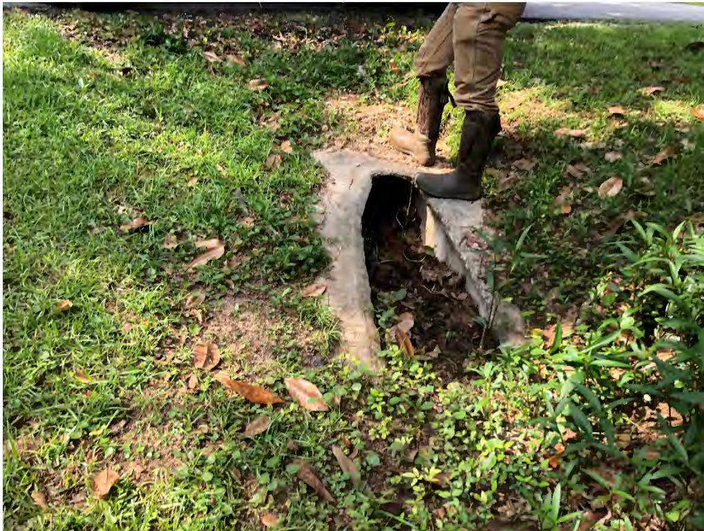
Figure 9256: Photo taken facing North toward P-CO-14 at the intersection of Pecan Grove St and Short Ave.
