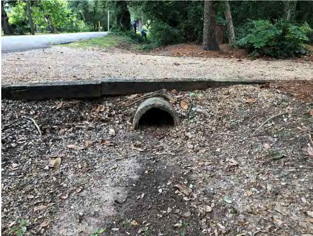
Figure 9145: Photo taken facing West toward a silted P-CO-20 along Oak St.
