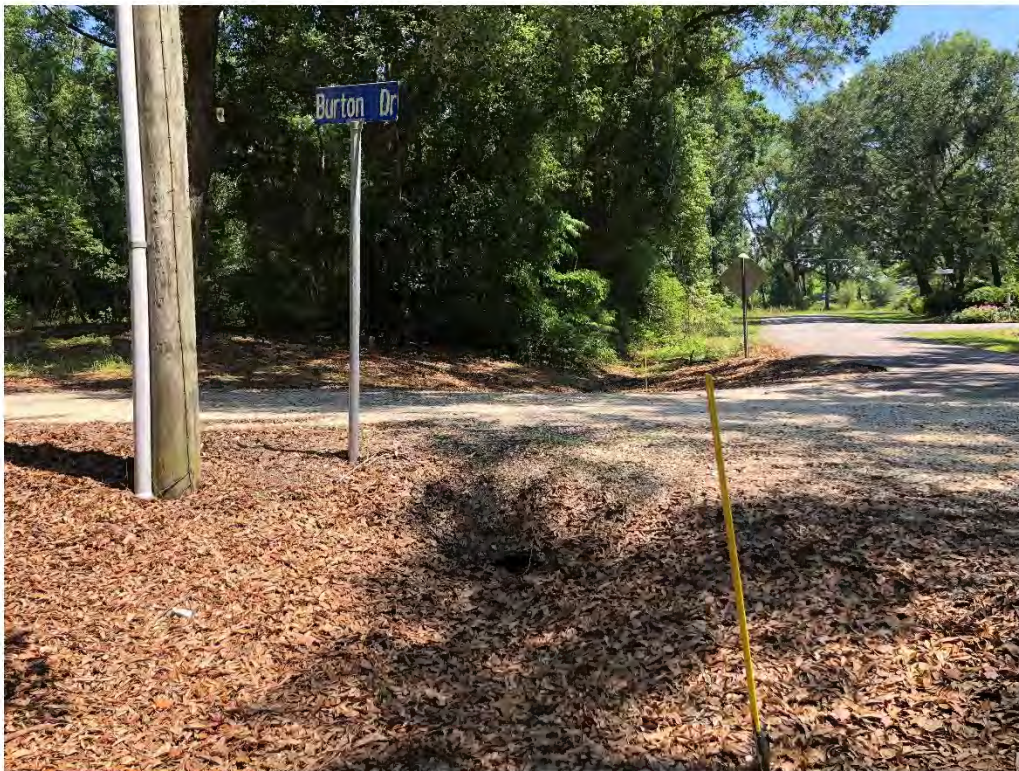
Figure 9038: Photo taken facing North toward a silted W-CO-2 at the intersection of Woodland Ave and a driveway.
