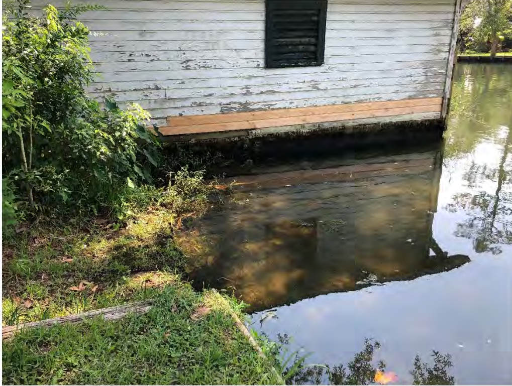
Figure 9643: Photo taken facing SE toward CH-200 along Jessamine St.
