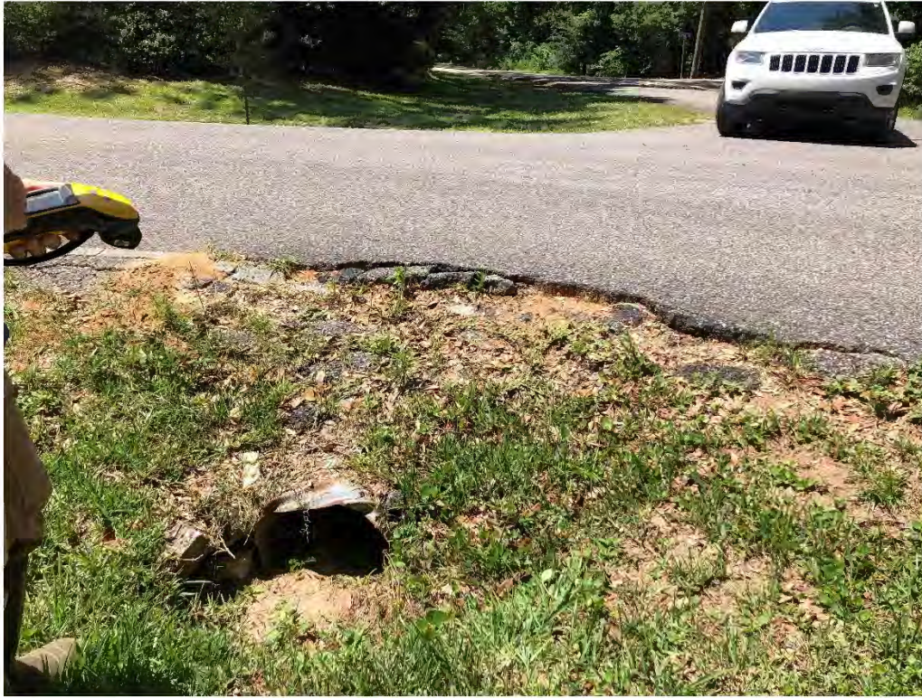
Figure 9046: Photo taken facing South toward a silted W-CO-1 at the intersection of Woodland Ave and Oak St.
