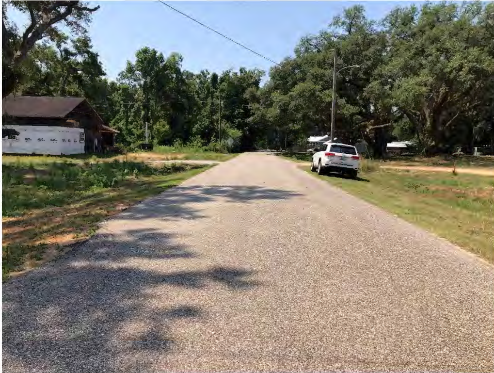
Figure 9619: Photo taken facing South toward OAK-CH-8 at the intersection HWY 98 and Jessamine St.
