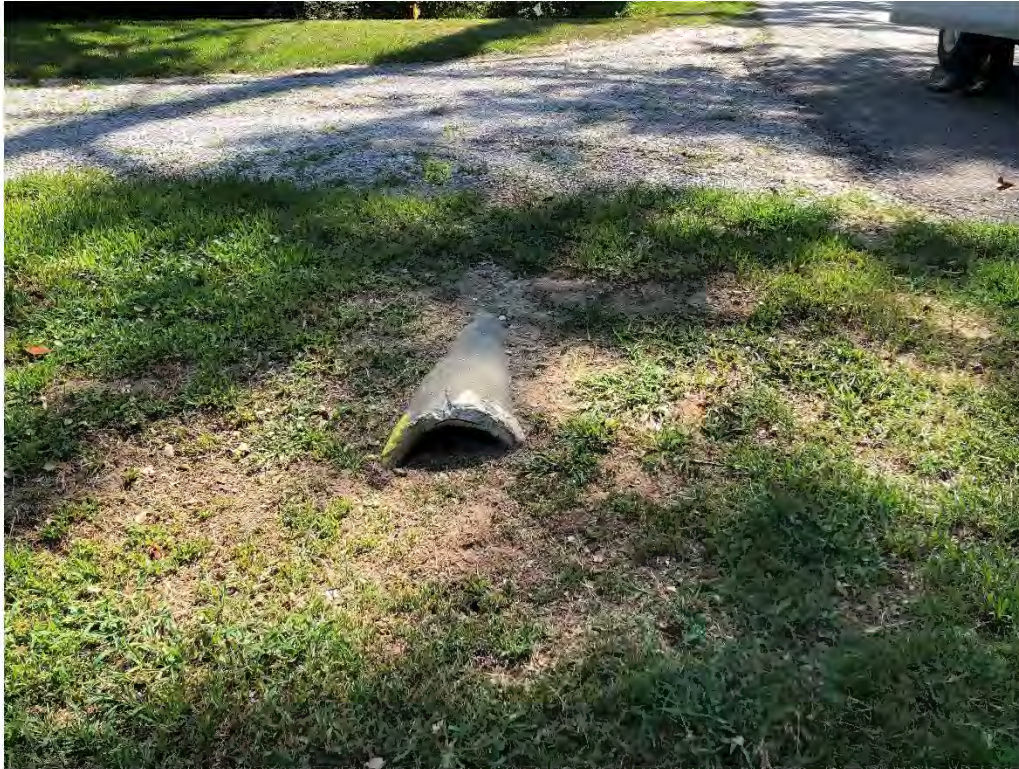
Figure 9523: Photo taken of a pipe across a residential driveway along Cotton Stocking Lane.
