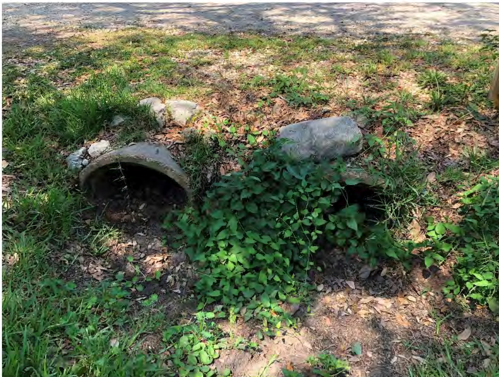
Figure 9606: Photo taken facing West toward a silted MN-CO-21 across a driveway.
