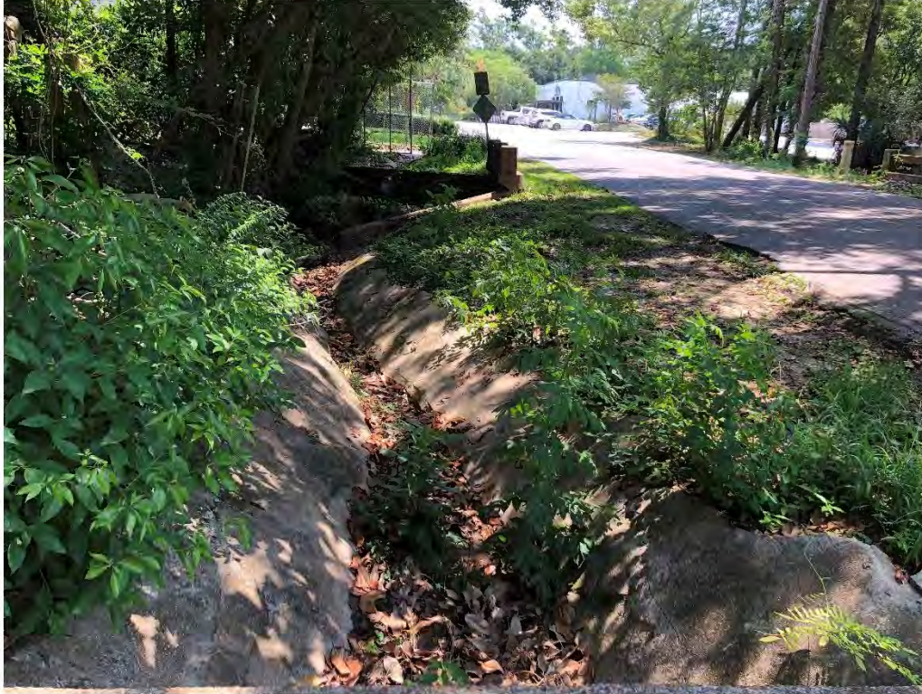
Figure 9666: Photo taken of a concrete ditch with moderate debris along Oak St.
