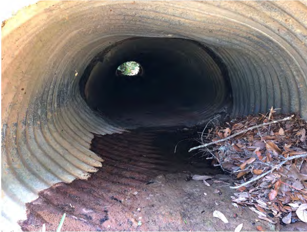
Figure 9110: Photo taken facing West toward a crushed corrugated metal P-CH-28 along Oak St.
