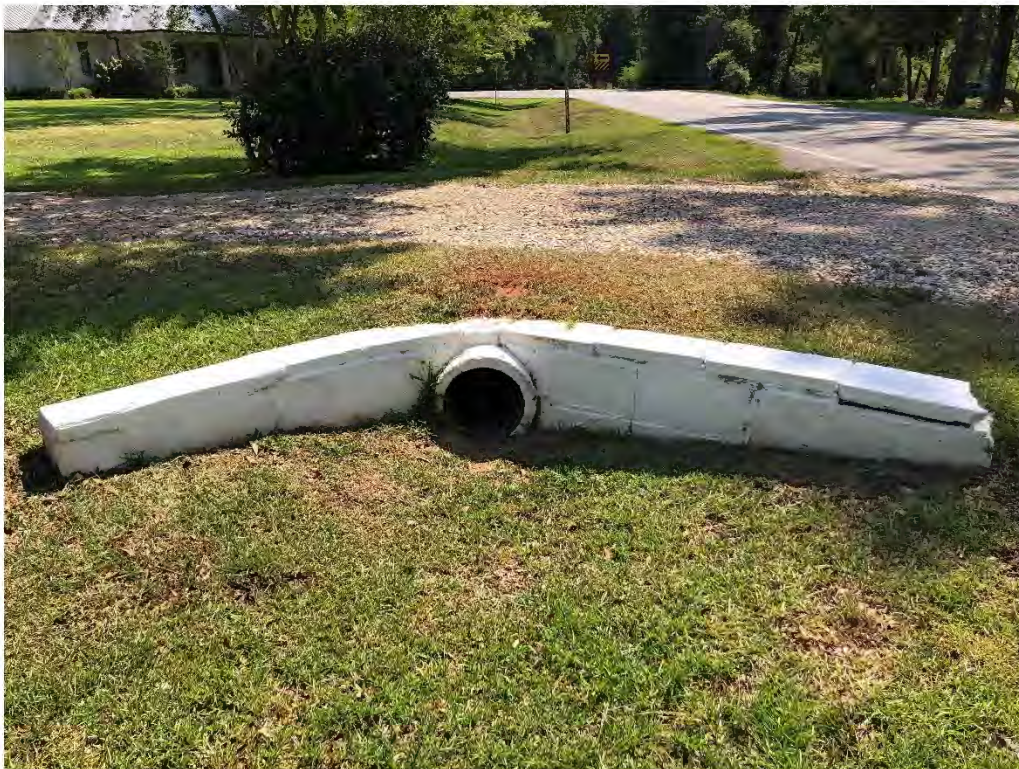
Figure 9562: Photo taken facing West of MN-CO-10 at the intersection of Gates Ave and a driveway.
