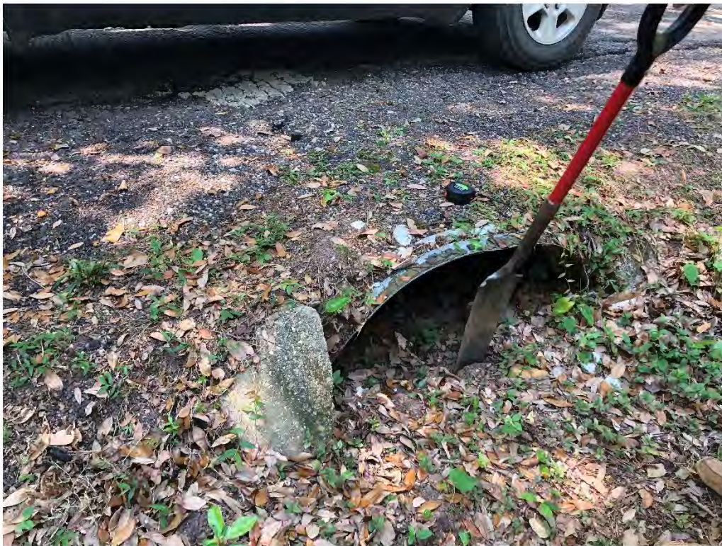
Figure 9646: Photo of a silted OAK-CO-18 that crosses McCoy Ln.
