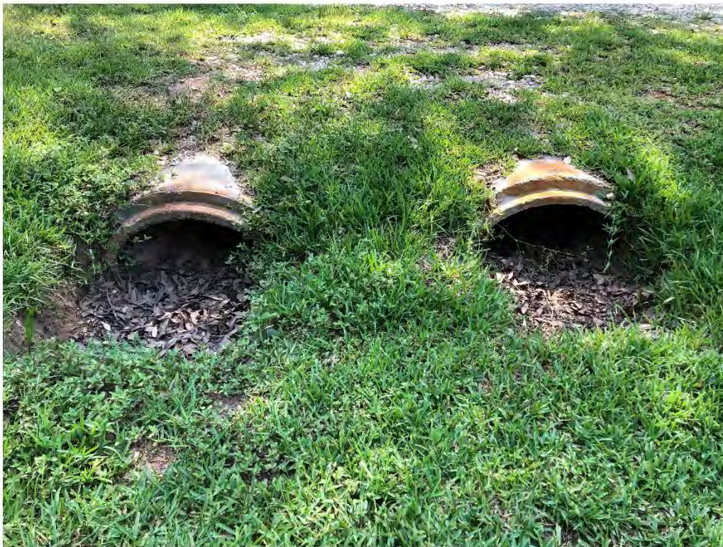
Figure 9608: Photo taken facing East toward a silted MN-CO-21 across a driveway.
