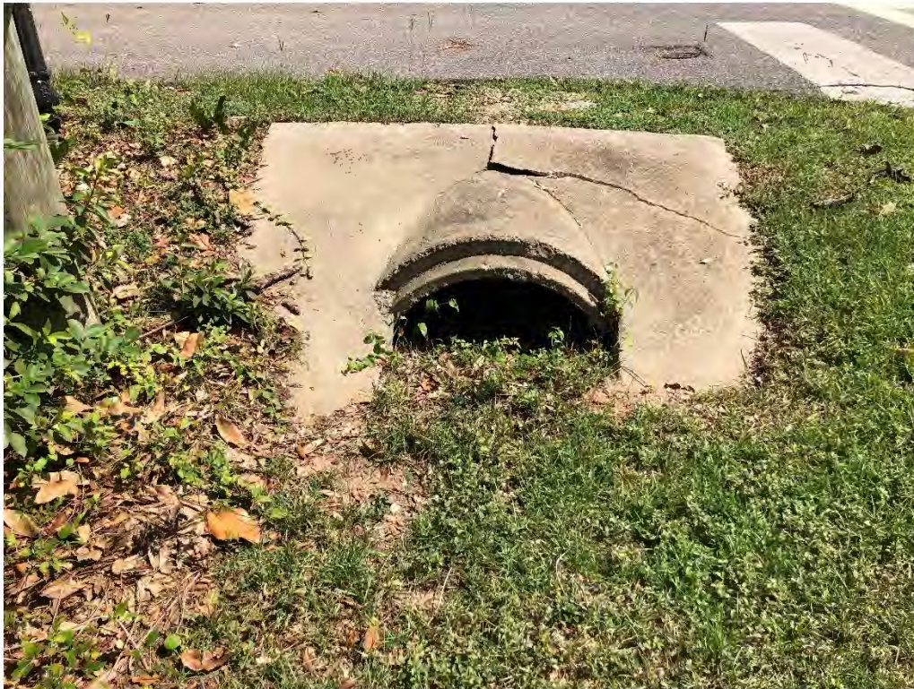
Figure 9547: Photo taken of OAK-CO-31 at the intersection of HWY 49 and School Street.
