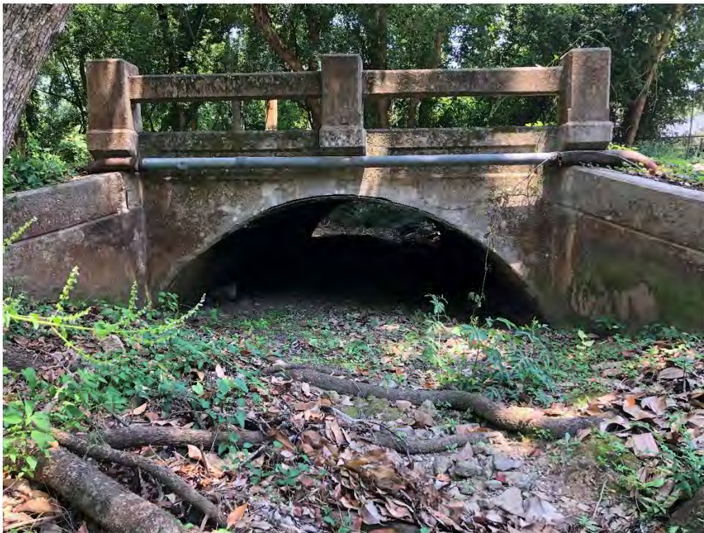
Figure 9675: Photo taken facing North toward a very silted OAK-CO-27 along Oak St.
