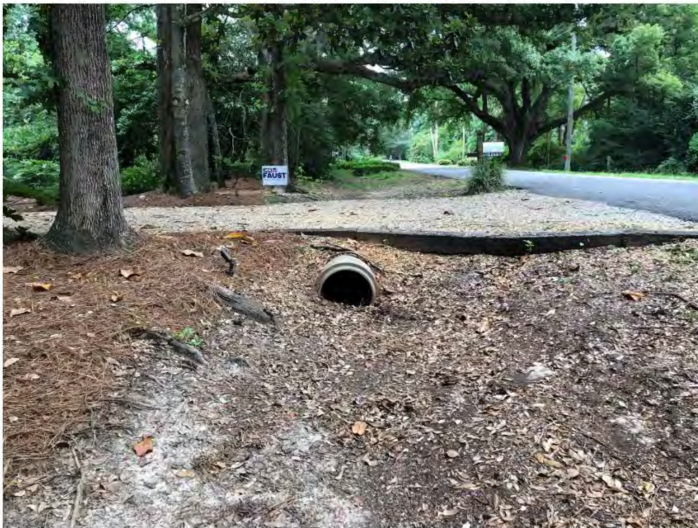
Figure 9144: Photo taken facing East toward a silted P-CO-20 along Oak St.
