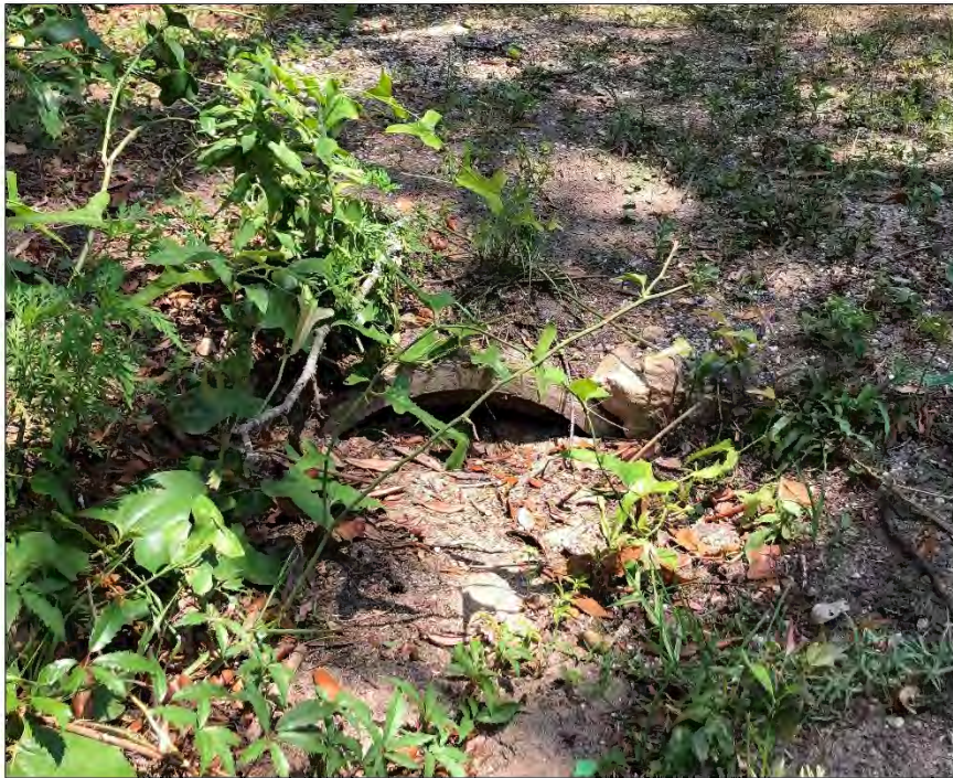
Figure 2. General view of sediment accumulation blocking pipe.
