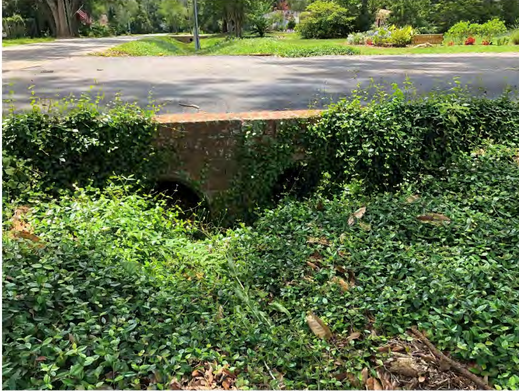
Figure 9120: Photo taken facing West toward an overgrown P-CO-24 along Oak St.
