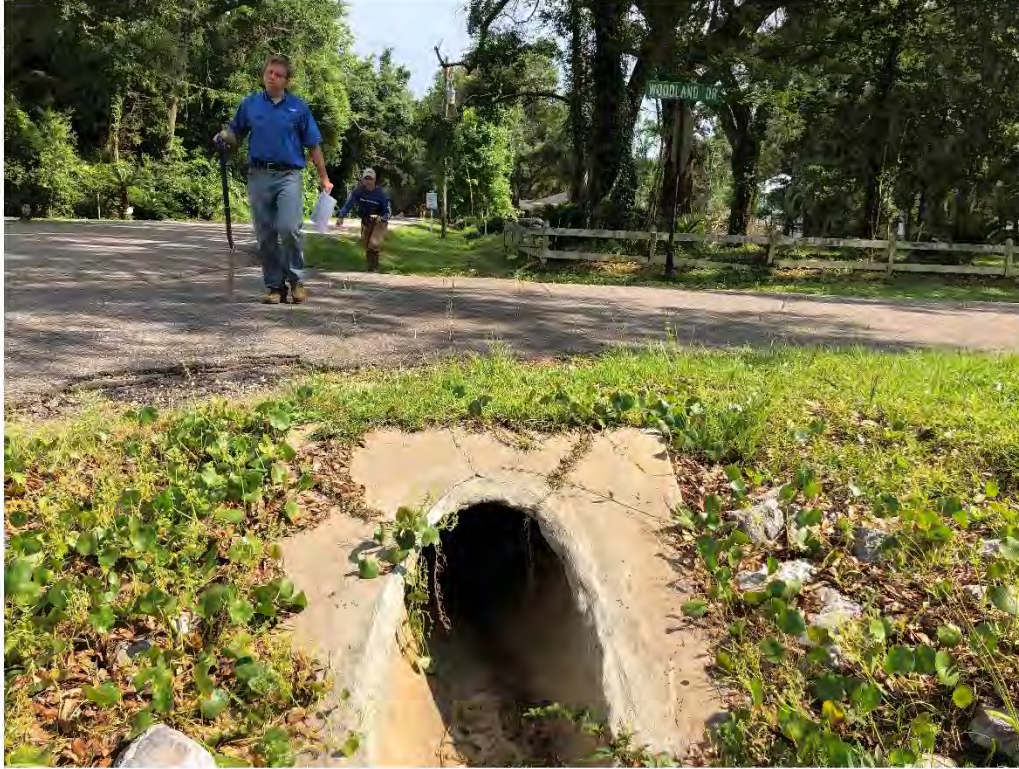
Figure 9248: Photo taken facing South toward P-CH-18 at the intersection of Pecan Grove St and Woodland Ave.
