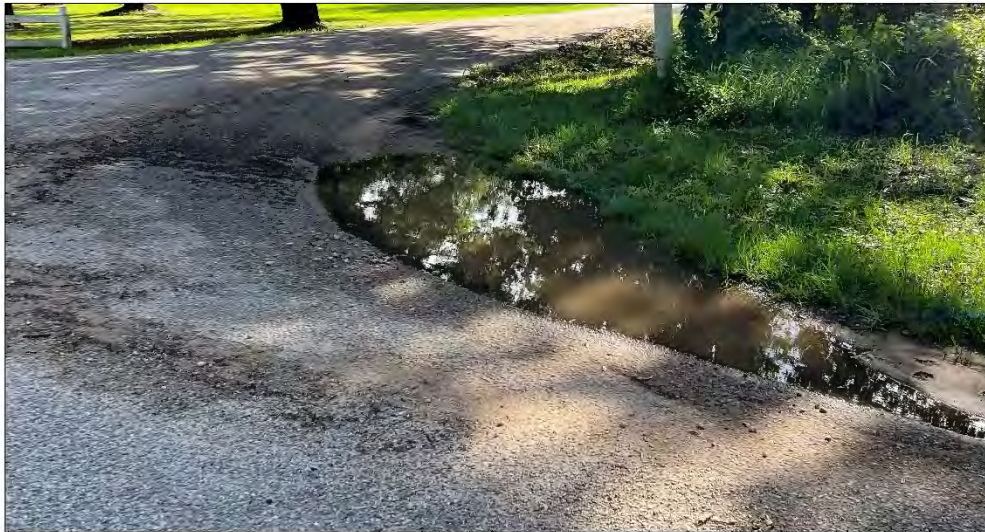
Figure 5. General view of standing water.
