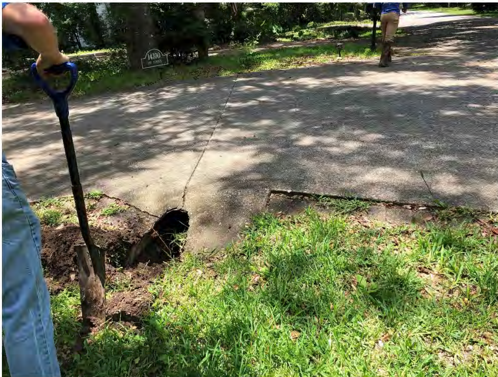
Figure 9075: Photo taken of a small, silted pipe along Oak St.
