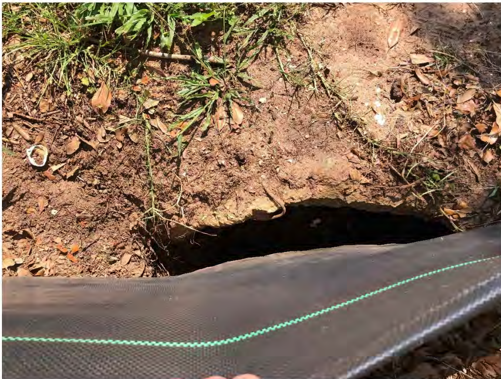
Figure 9626: Photo taken facing East toward a crushed and very silted OAK-CO-6 across Jessamine St.
