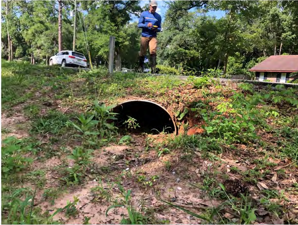
Figure 9243: Photo taken facing SW toward a silted P-CO-17 along Pecan Grove St.
