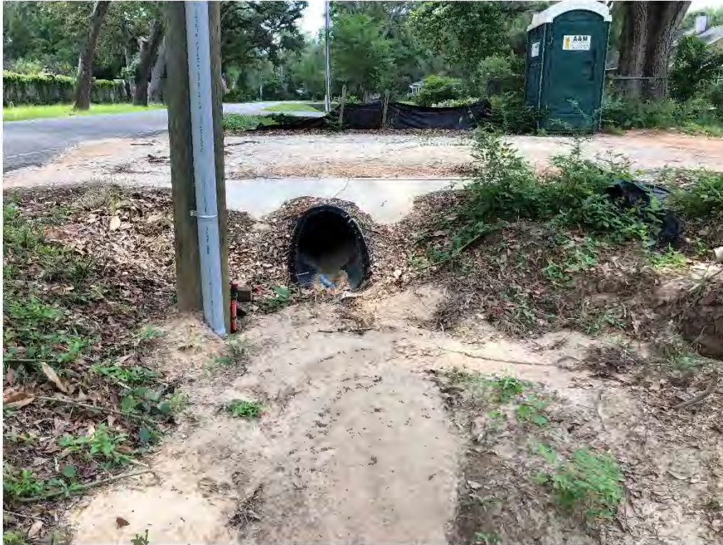
Figure 9126: Photo taken facing West toward a silted P-CO-23 along Oak St.
