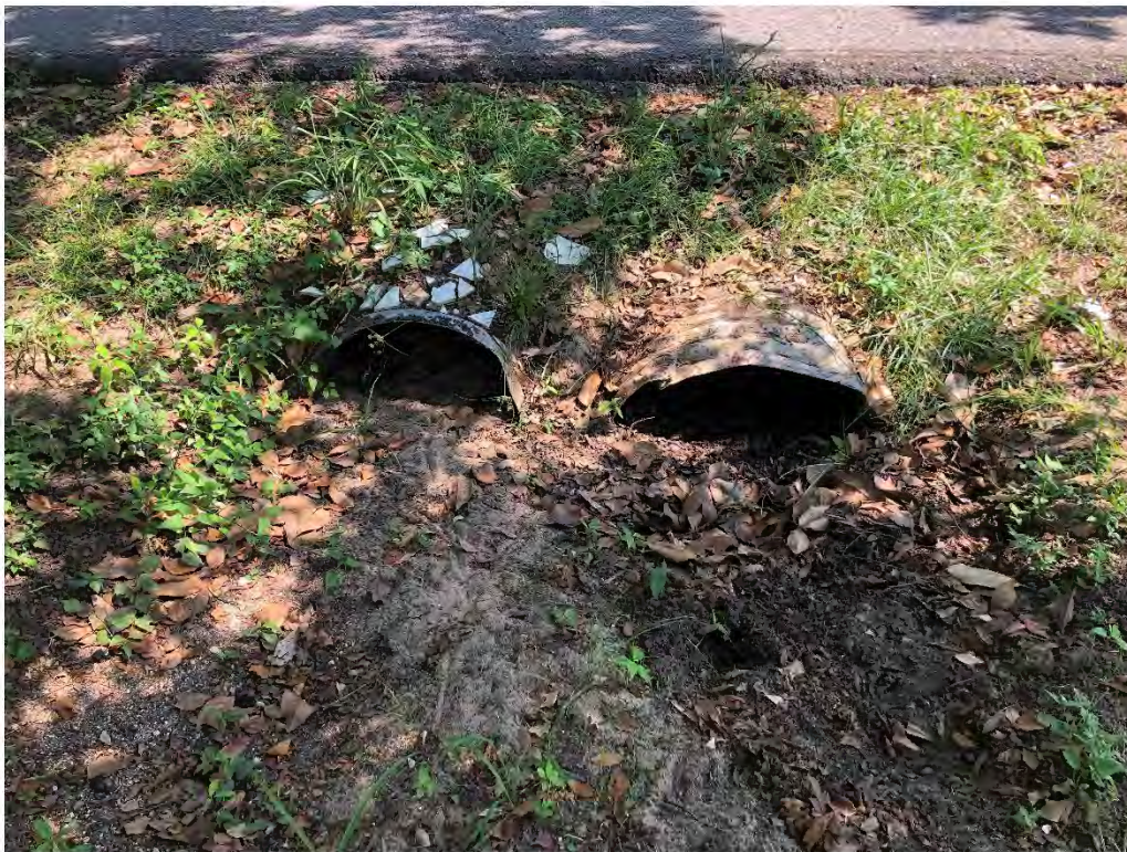
Figure 9598: Photo taken of a silted pipe at the intersection of School Street and Magnolia Ave.
