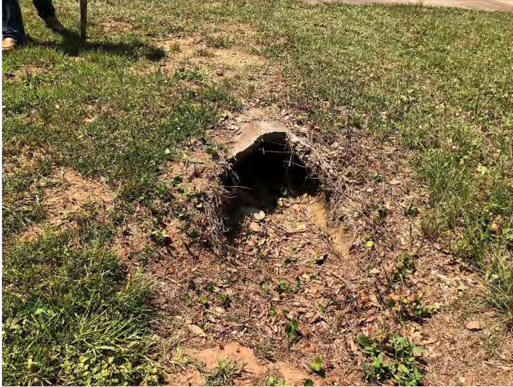
Figure 9637: Photo taken facing South toward a silted OAK-CO-9 that crosses Jessamine St.
