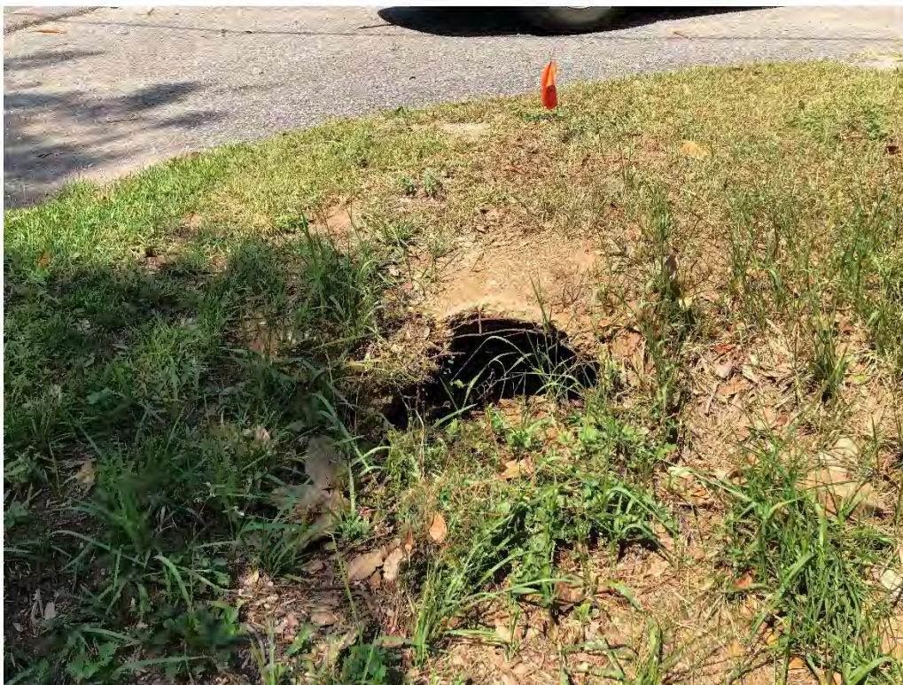
Figure 9573: Photo taken facing West of MN-CO-14 at the intersection of Gates Ave and a driveway.
