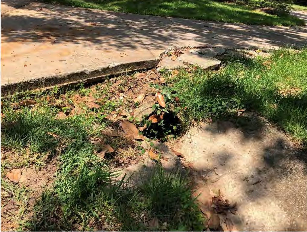
Figure 9661: Photo taken facing SW toward a concrete ditch that is full of dirt along Oak St.
