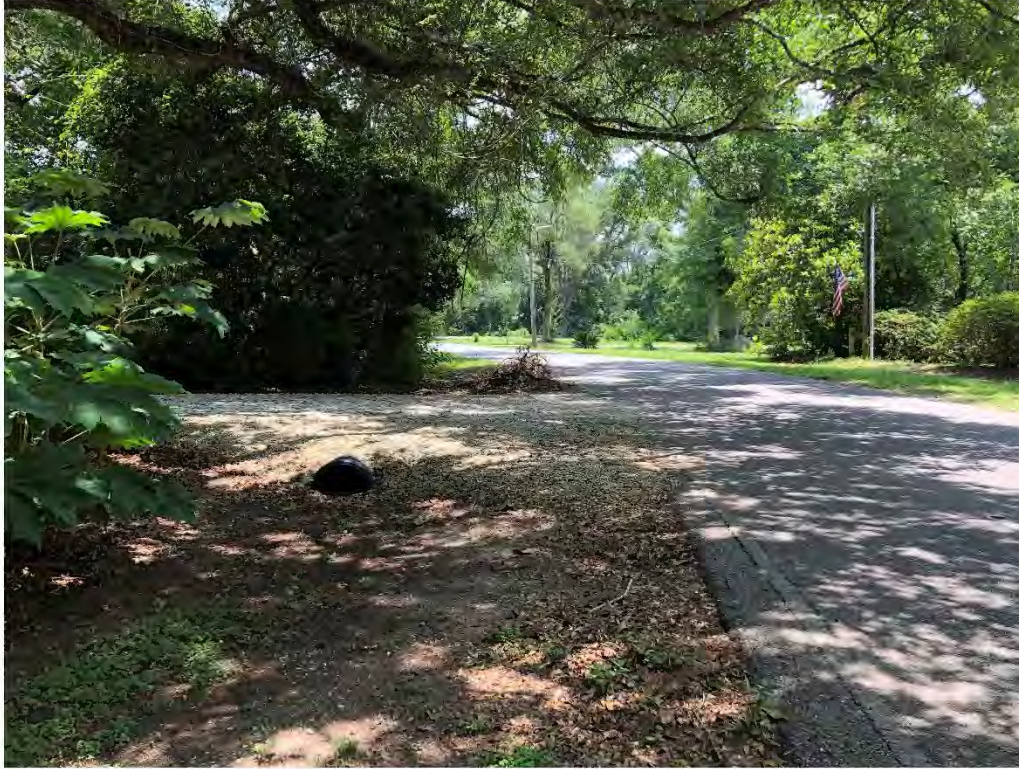
Figure 9078: Photo taken facing East toward a silted P-CO-25 along Oak St.
