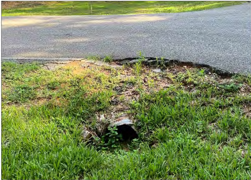
Figure 3. General view of asphalt edge raveling.
