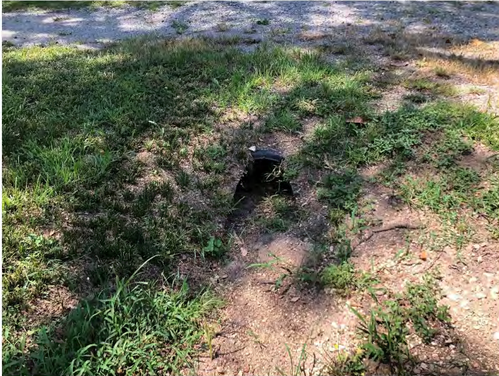
Figure 9603: Photo taken of a pipe at the intersection of School Street and a driveway.
