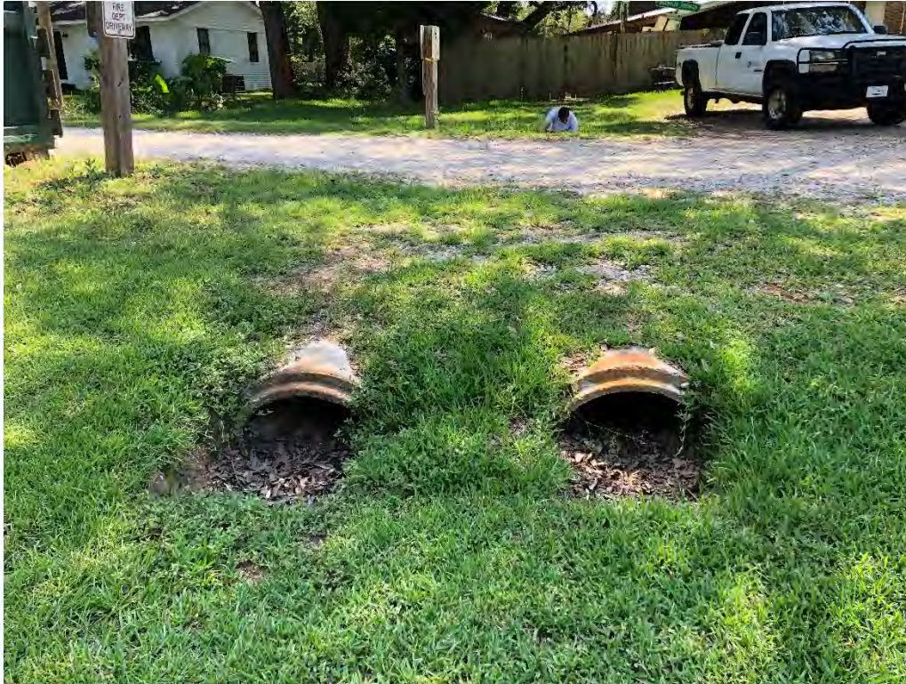
Figure 9607: Photo taken facing East toward a silted MN-CO-21 across a driveway.
