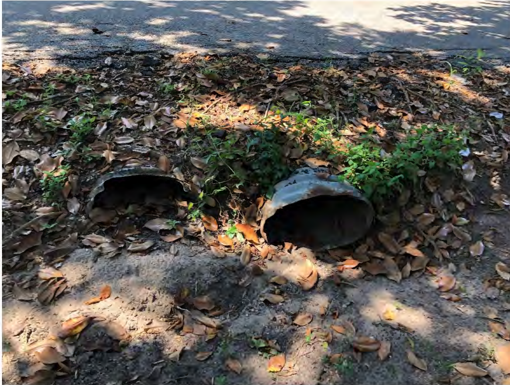
Figure 9599: Photo taken of a silted pipe at the intersection of School Street and Magnolia Ave.
