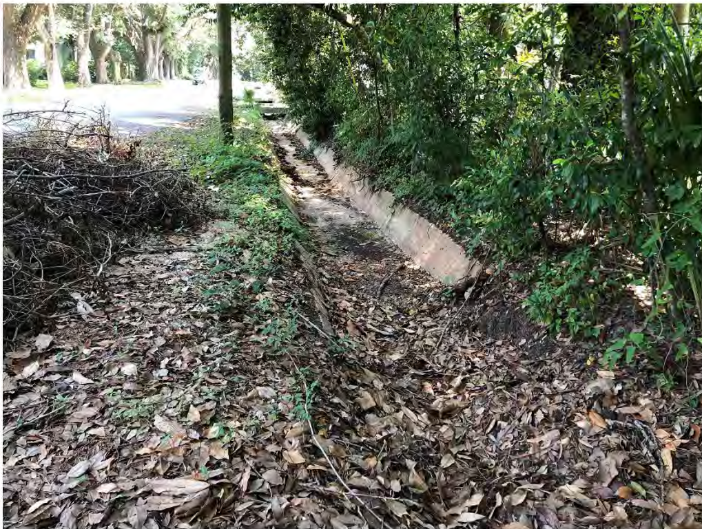
Figure 9642: Photo taken facing North toward a concrete CH-200 with moderate debris along Jessamine St.
