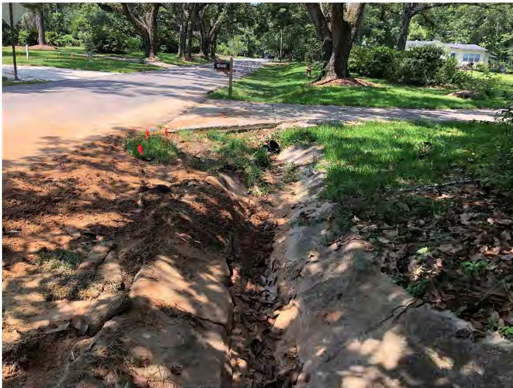
Figure 9660: Photo taken facing SW toward a concrete ditch that is full of dirt along Oak St.
