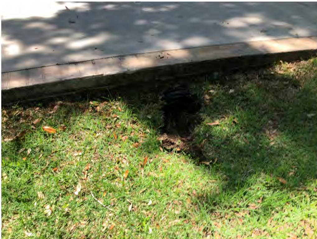
Figure 9060: Photo taken facing West toward a damaged P-CO-29 along Oak St.
