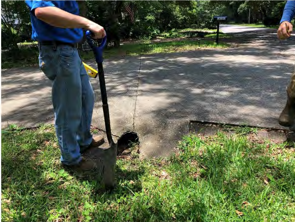
Figure 9074: Photo taken of a small, silted pipe along Oak St.
