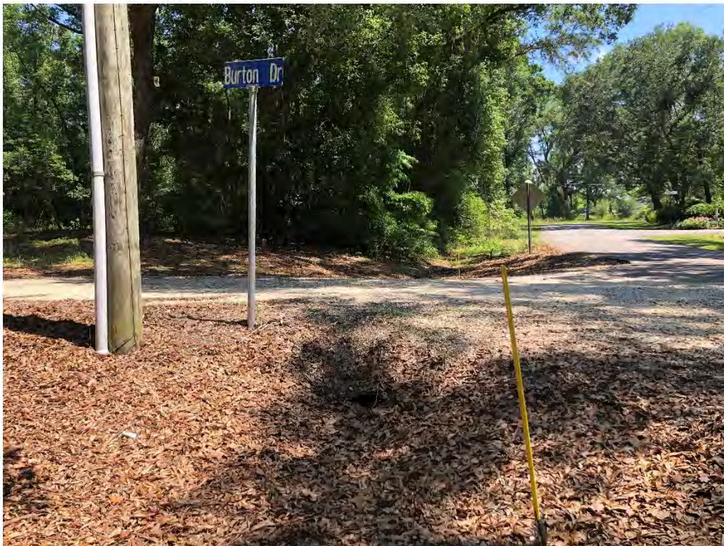
Figure 9038: Photo taken facing North toward a silted W-CO-2 at the intersection of Woodland Ave and a driveway.
