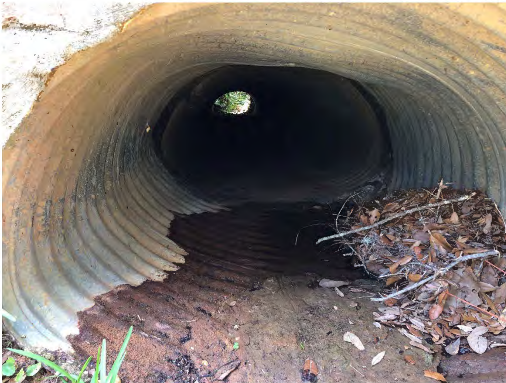
Figure 9111: Photo taken facing West toward a crushed corrugated metal P-CH-28 along Oak St.
