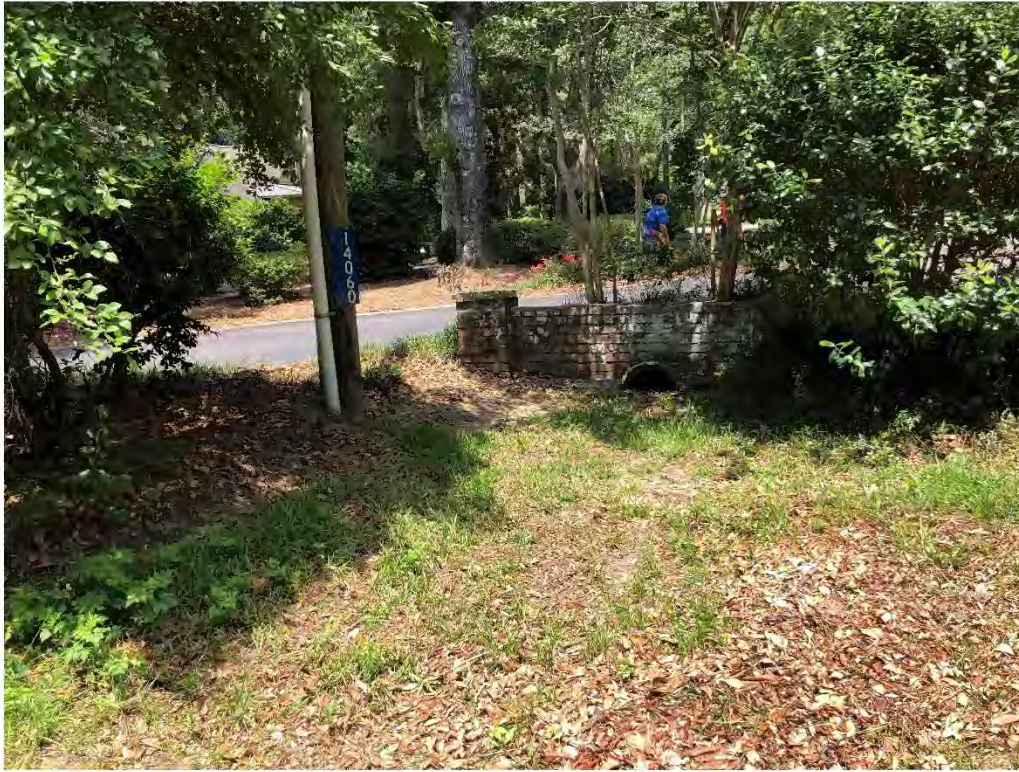
Figure 9071: Photo taken facing West toward a silted P-CO-32 along Oak St.
