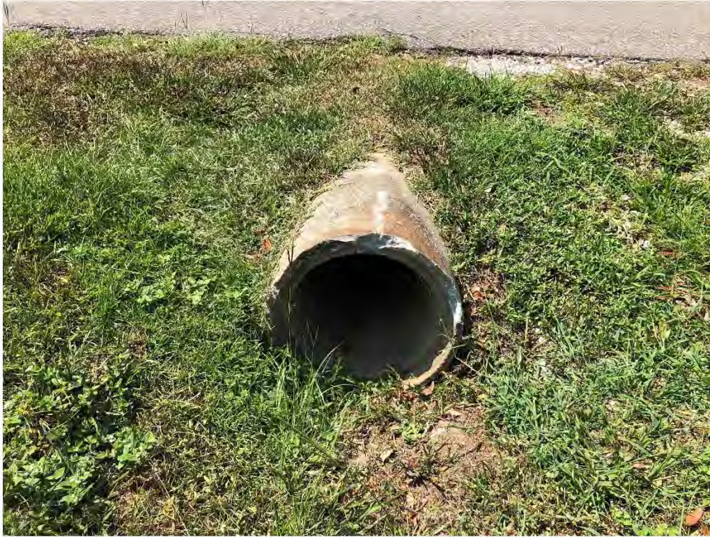
Figure 9615: Photo taken facing South toward a silted MN-C0-3 at the intersection HWY 49 and a driveway.
