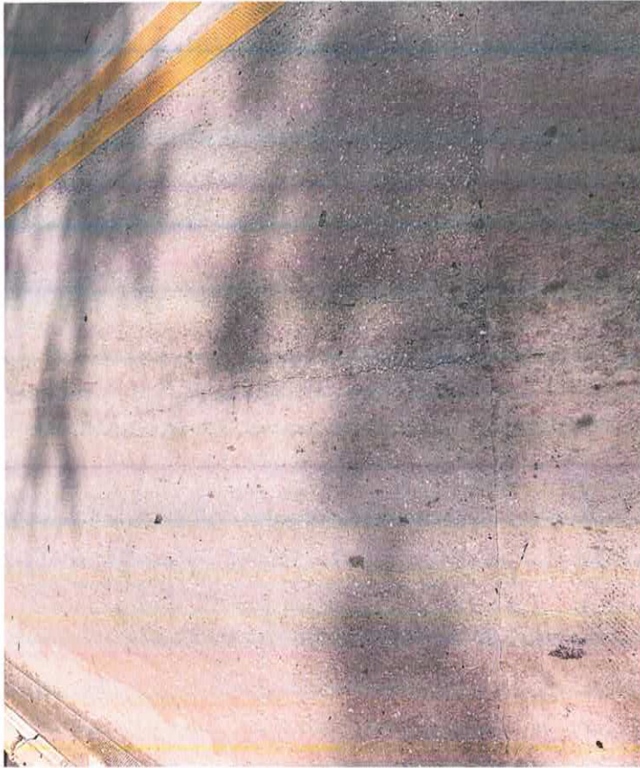
CS3 crack on deck
