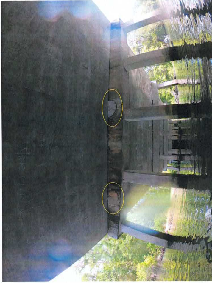
Bent 5 patch and spall
