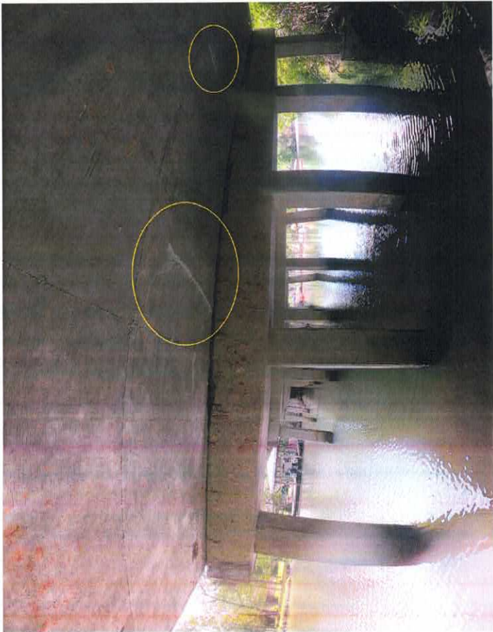
Eff on ceiling
