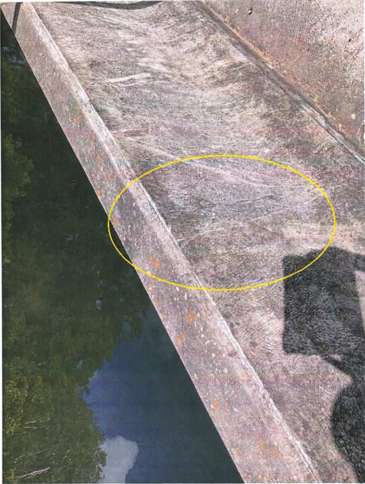
Hairline cracking on concrete railing
