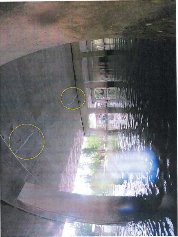
Eff on ceiling (2)
